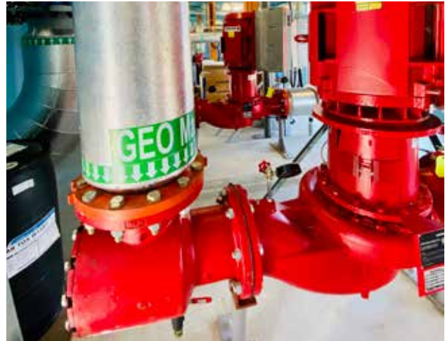
The Alexandra District Energy Utility distribution pumps disburse thermal energy through the underground pipe network.
